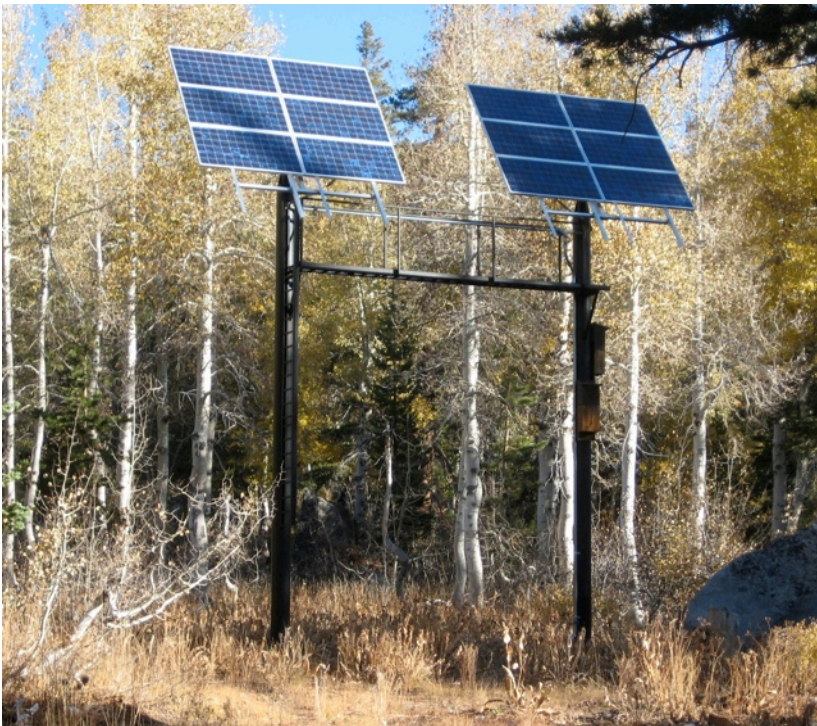
Solar Panels Near Kirkwood
